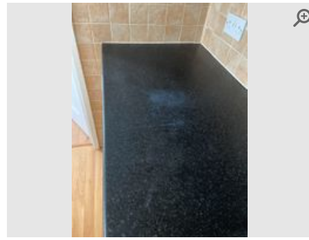
Provided by Inspector Captured (via App): 04/02/2020 12:47 PM Added 04/02/2020
